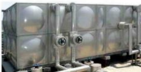
Industrial Water Tank
