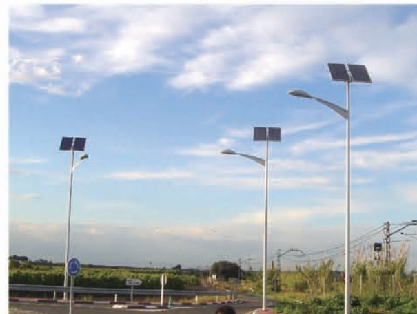
Solar street lamp in Spain
