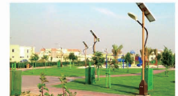
A solar street lighting system in Dubai
