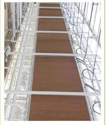
湿帘墙用于温室大棚 Cooling Pad Wall used in Greenhouse
